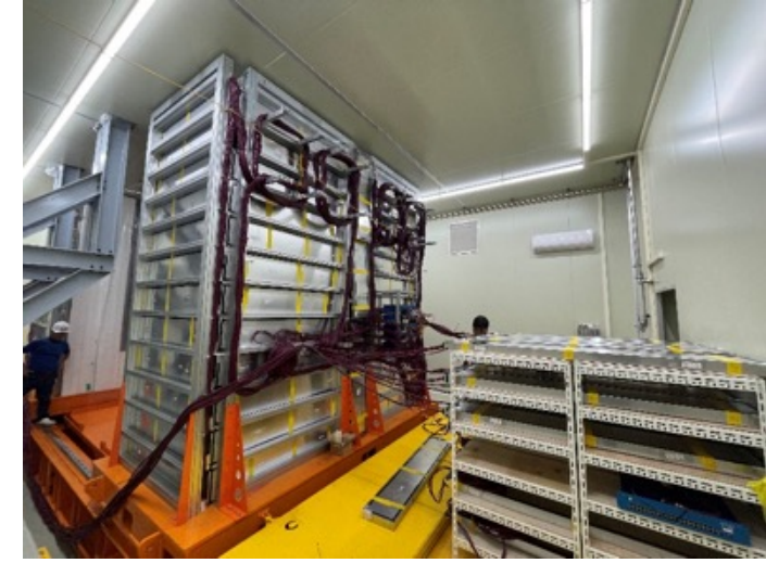
AMoRE-II • Shield structure done • Late 2024, commissioning
